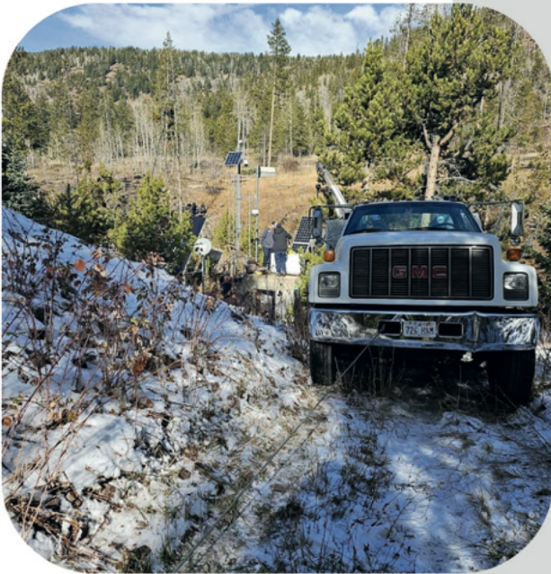
Installation of the new generator at the Duchesne Tunnel Outlet measuring station
